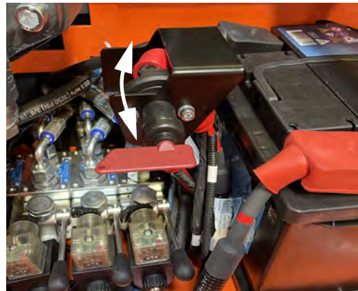
BATTERY DISCONNECT SWITCH
